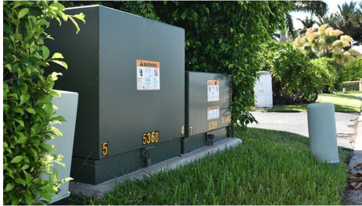
Figure 12 Underground Pad-Mounted Transformers 2026
